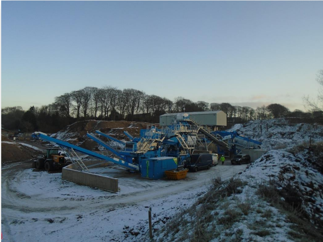
Wash plant as built
